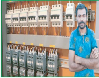
ELECTRICAL PANEL BOARD
