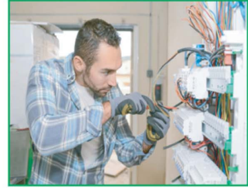
ELECTRICAL SWITCHED BOARD
